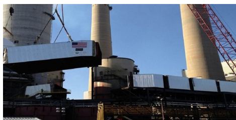
Graycor Industrial Constructors completed a wet flue gas desulfurization system at NIPSCO's R.M. Schahfer Generating Station located in Wheatfield, Ind., in 2014. Source: Graycor
